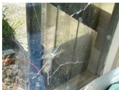
#34: Broken window. Lounge northern wall.
