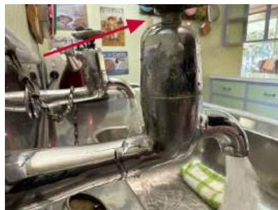
#48: Hot water tap leaking when in use.
