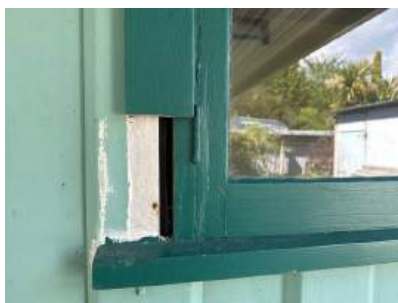
#105: Laundry window is missing part of the facing board
