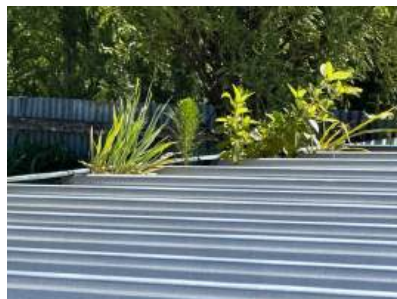
#238: vegetation in gutter, cleaning is recommended
