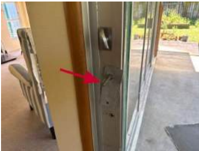
#39: missing handle dining room
