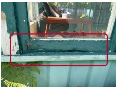
#107: Timber decay. Lounge western window.
