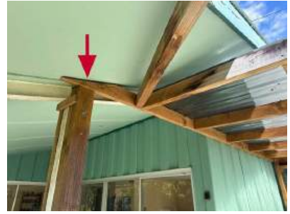
#113: improvement to the support at the end of the verandah is recommended.
