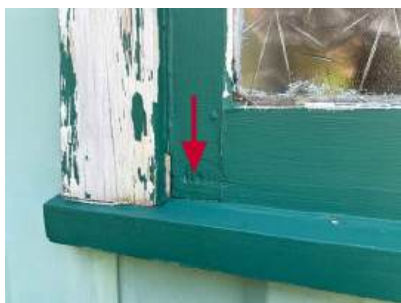
#104: Timber decay to toilet window.
