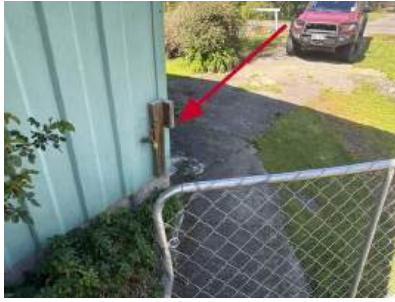
#249: gate latch attached to cladding
