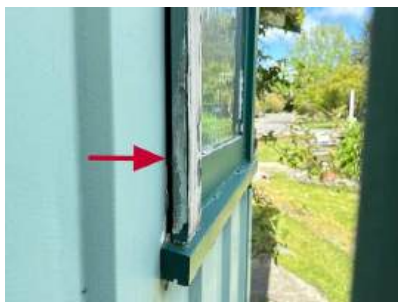
#108: Gaps at cladding junctions
