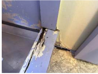
#69: timber decay to the shower step
