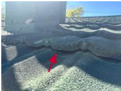
#128: lifted nail causing lap joints to be exposed
