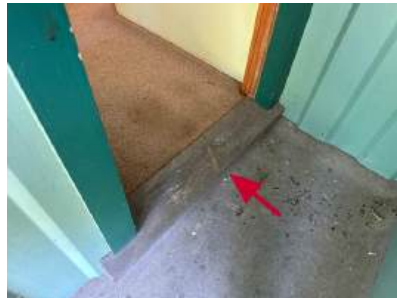
#40: door sill is loose
