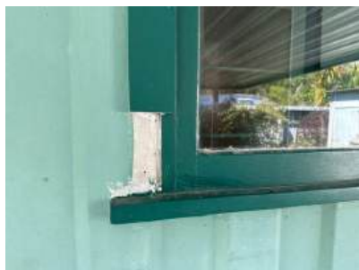
#106: Entrance window is missing part of the facing board.
